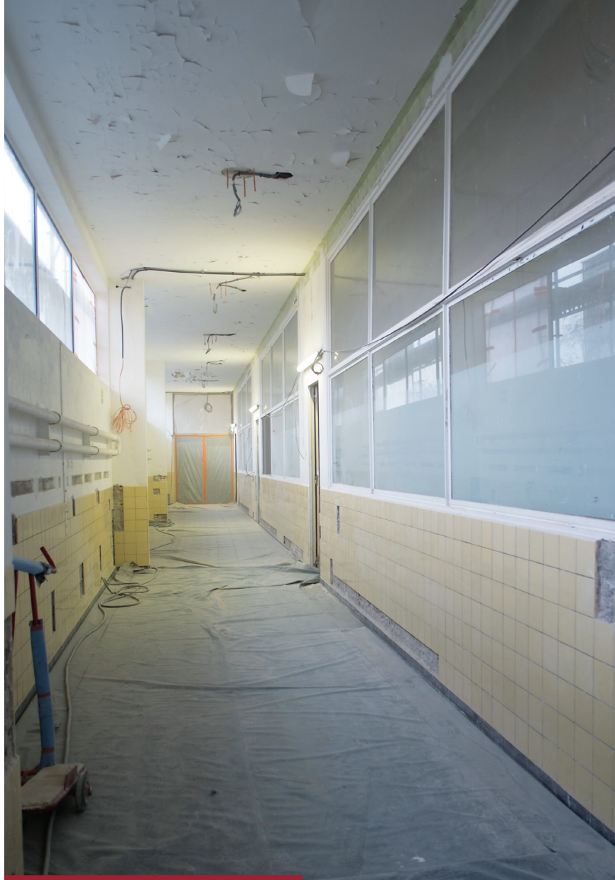
The school's hallway during construction (left) and after intervention (right). Ninety percent of the glazed ceramics covering the walls were preserved.
