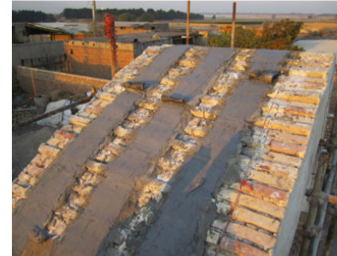
22. Epoxy mortar applied onto base layer, with glass fibre mesh embedded between two layers of the mortar.
