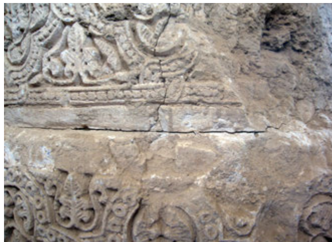
3. Horizontal crack in column 11.
