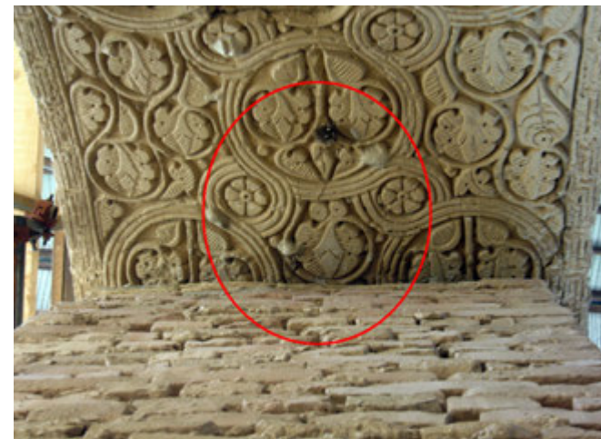
4. Supported arch intrados: the start of the inner fracture (due to torsional component). Arch 10–11.
