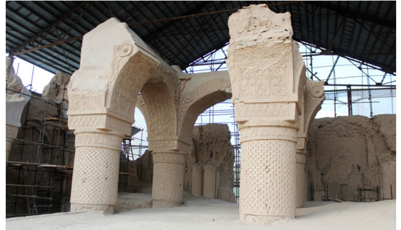
108. General view of the arch system (6-10 and 10-11) looking from north-east, after consolidation.
