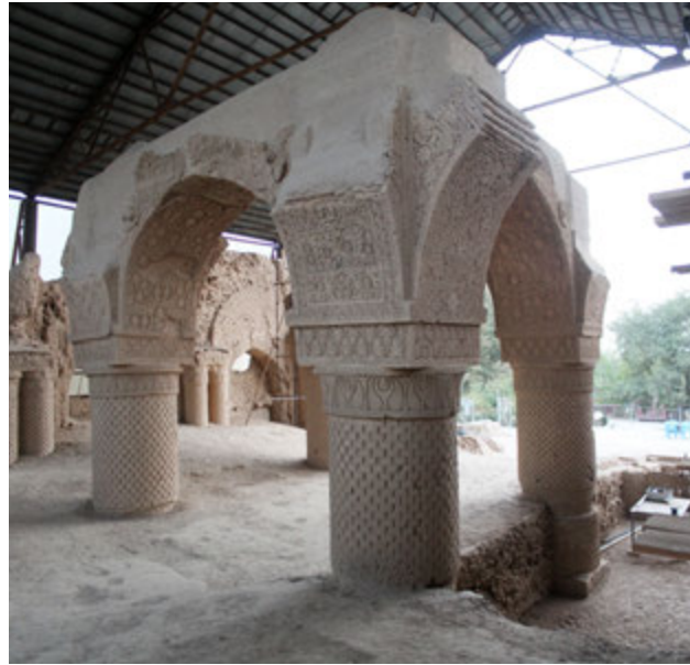
106. General view of the arch system (6-10 and 10-11) looking from South West, after consolidation.
