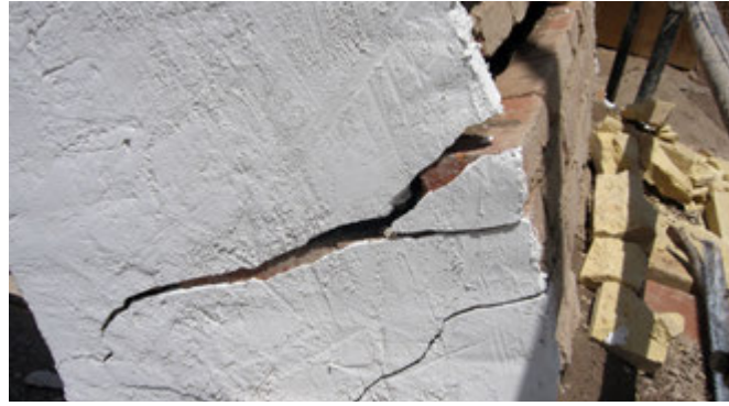
19. Cracks on the shoulder caused by the column base lifted by 3.7 cm or 1.14 degrees by hydraulic jacks.
